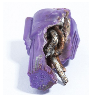
Corroded Al-Cu contact copper-electric.net
